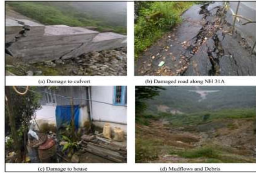
Observed damages during field visit (Dikshit and Satyam, IIS, 2018)
